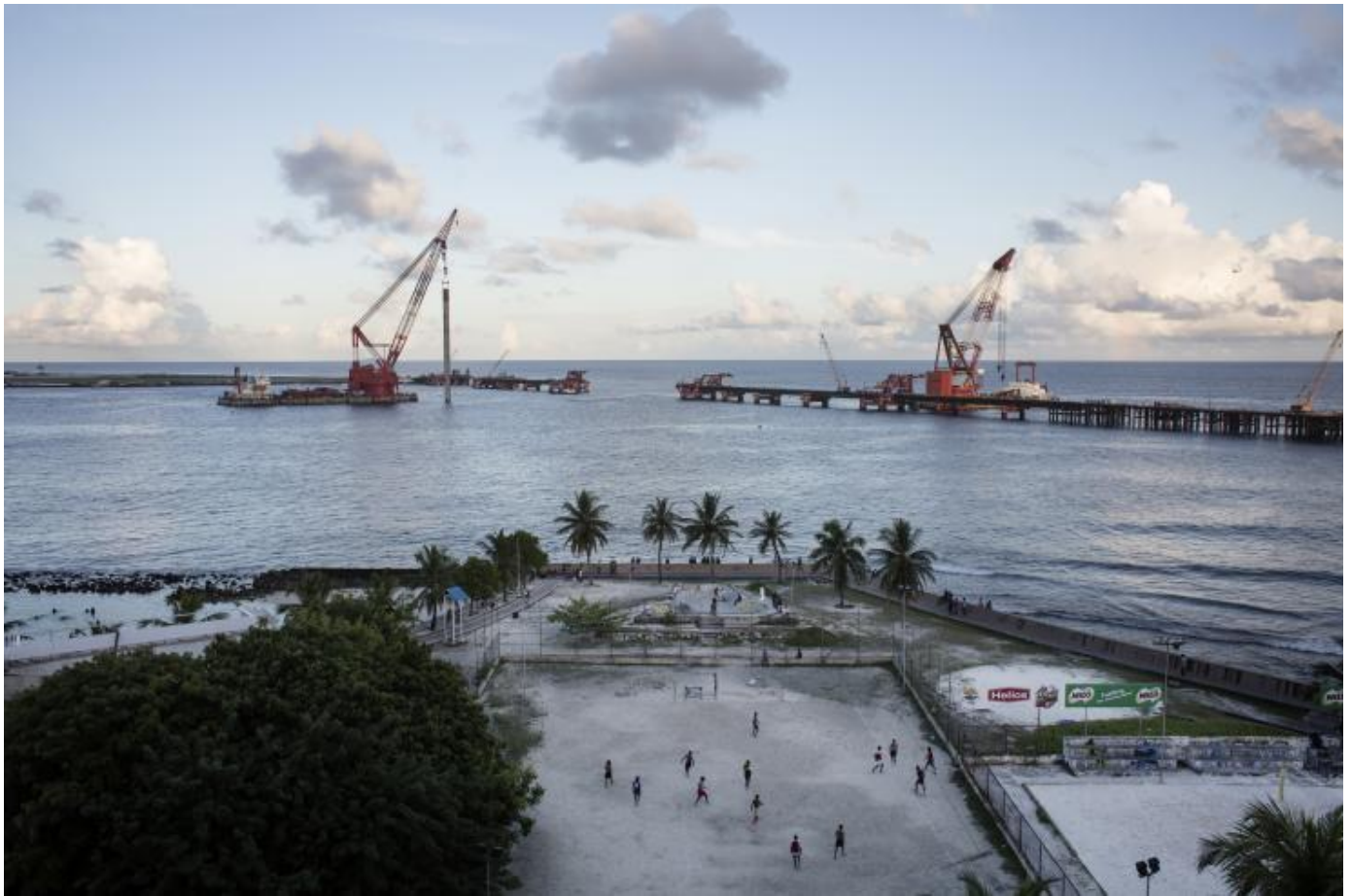
Bridge construction project connecting the capital island Male to the airport island of Hulhule on October 27, 2016 in Male, Maldives.
